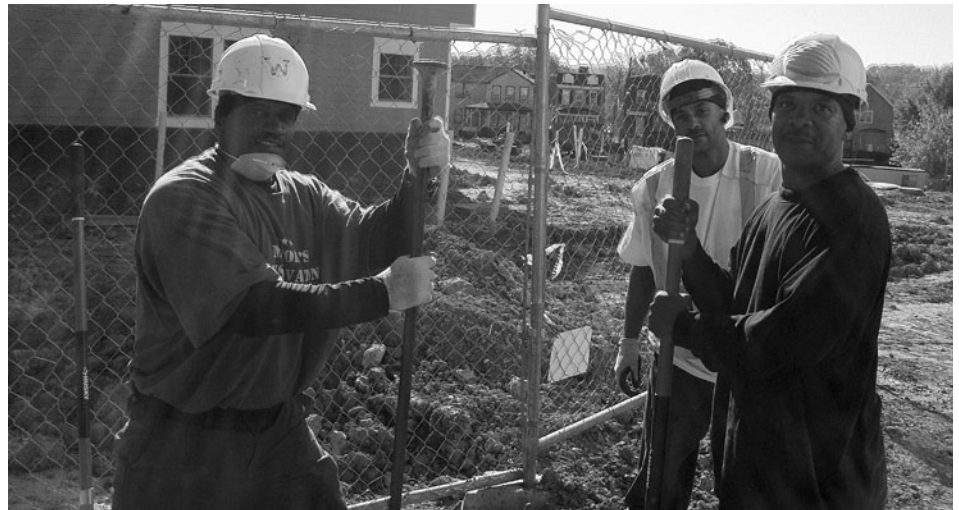
Community members hired to work on UrbanMatters development projects. Photo courtesy of Spence Limbocker.
